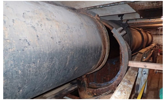
Figure 2: Failed Equalizer Pipe
