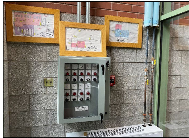
Smoke Evacuation Control Panel
