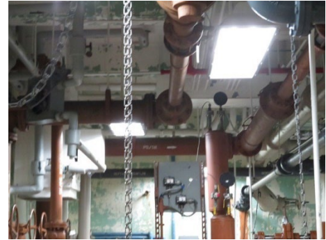
New LED Lights at Clinton Treatment Plant
