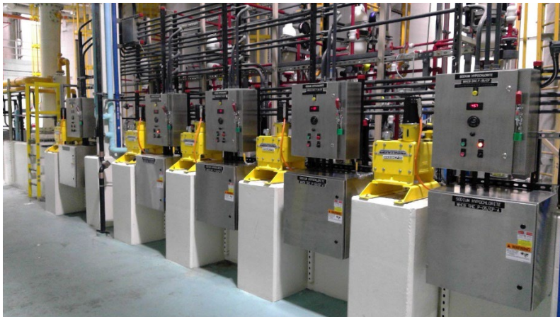
Sodium Hypochlorite Upgrades
